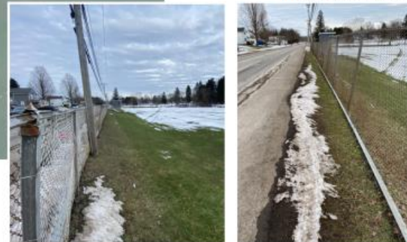
Proposed improvements will remove existing steel guiderail, chain link fence, and a portion of the paved shoulder.
